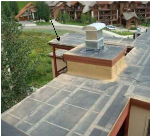
Recently installed elevator power ventilation unit. Photo shows temporary “ice and water shield” flashing between sheet metal vent and roof deck. This needs proper flashing.
