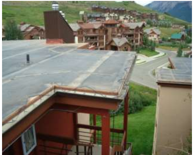
Roof Deck 2. Photo depicts snowmelt cable at roof edges and in rain gutters. This detail will be carried over into the replacement roofing.
