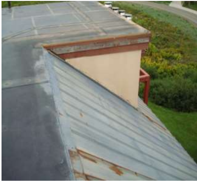
Weathered wood fascia and trim. Re-staining should be performed soon. Also, photo depicts aged metal deck.
