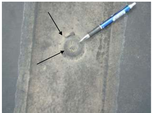
Round spots are the EPDM over fasteners that attach underlayment board to the roof deck. Cracking and small cuts are depicted in this photo at the tip of the arrows. They are about a 1/4" in length.
