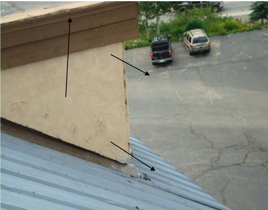
NW corner of upper roof deck. Photo attempts to depict a condition where the stucco at the corner is deteriorated to the point that water could penetrate (lower arrows). Attempts have been made to seal the stucco on these corners. Likewise, the seal between the edge metal and EPDM is starting to deteriorate (top arrow). Due to steepness of metal roof deck, unable to closely inspect the vertical corner or flashing. The metal roof deck appeared to be in fair condition.
