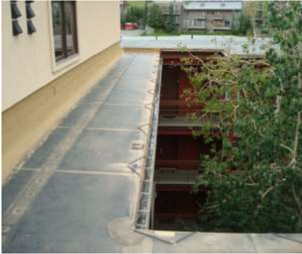
Photo depicts snowmelt cable at eaves and rain gutters. Shown in PHOTO 11 below is “checking” in the EPDM surface. This was noted in this area.
