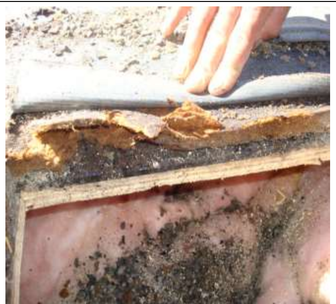
Same location as photo 23. Photo depicts EPDM pulled back, underlayment board, gravel, asphaltic material, plywood and insulation. The underlayment is wet. The underside of plywood, insulation and 2x12 joist are dry.
