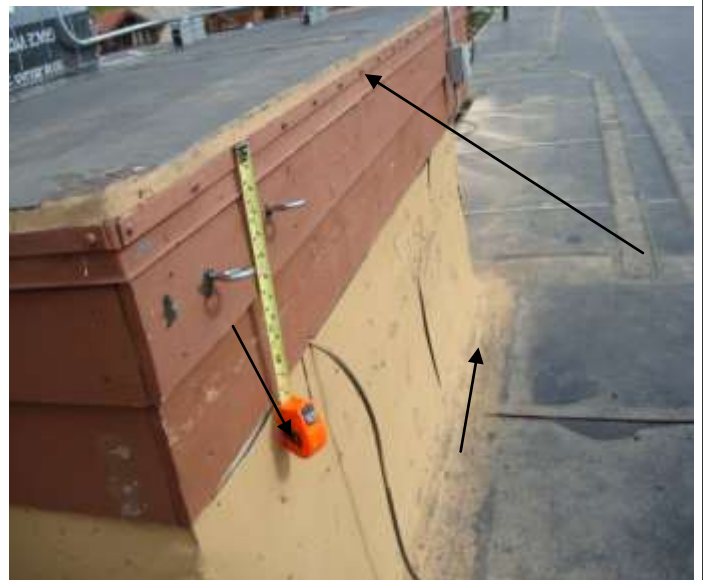
Photo shows loose flashing below wood fascia. Also, metal edging with exposed fasteners. Single ply roofing manufactures today still use the edge metal to hold the single ply along edges but the edge metal is sealed with an adhesive applied membrane strip. Fasteners and metal (termination bars) are not exposed in more modern installations.
