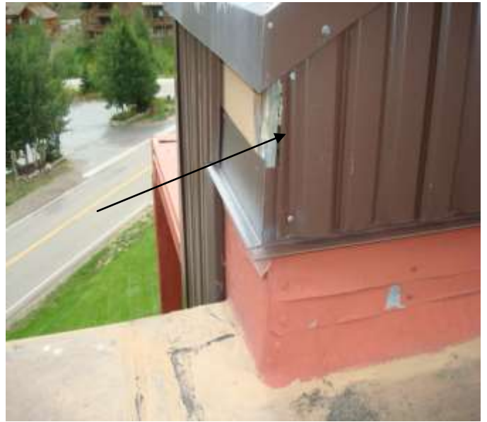
Corner flashing damage.
