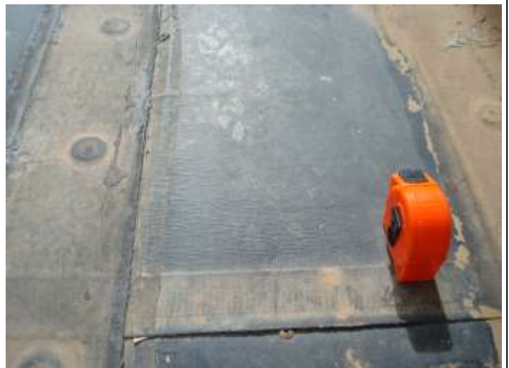
Photo depicts loose seam and checking. Checking is hard to see in the photo but is a sign of aging EPDM subjected to conditions prevalent in Mt Crested Butte. This area will be investigated to the wood deck.
