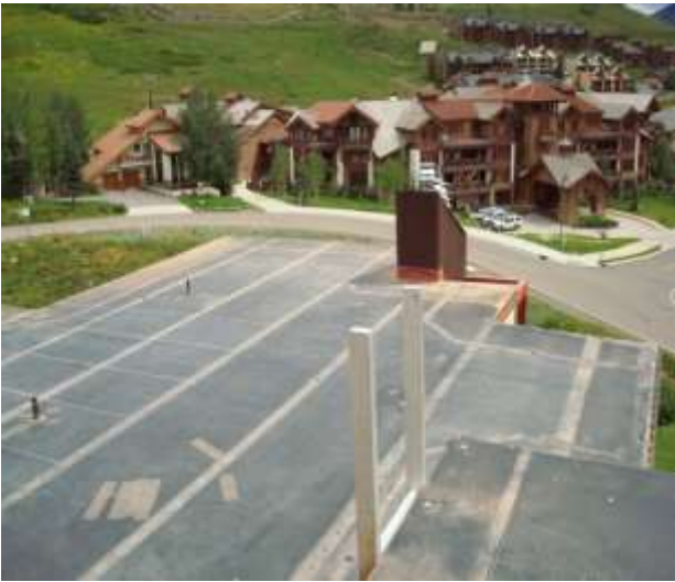
Overall photo of Roof Deck 2 from Roof Deck 1. Patching from previous repairs are visible.
