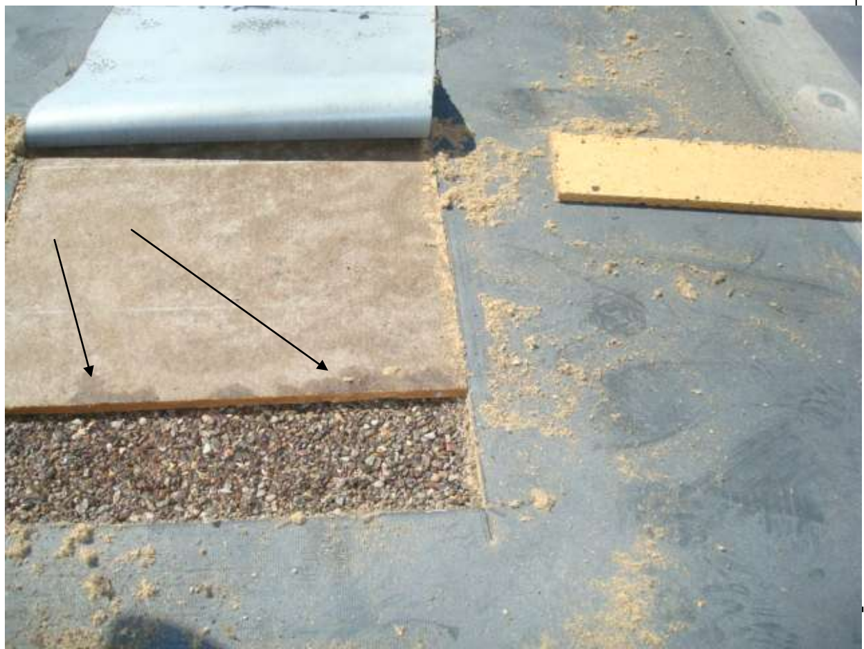
This is roof deck 2, at a location where no cuts or tears were visible. The underlayment and gravel was wet but not as saturated as locations where cuts were present. The dark areas on the underlayment is water brought up by the saw. The gravel in this photo is wet.
