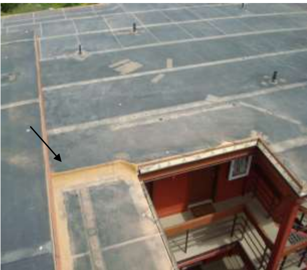
This photo shows Roof Deck 2 from Roof Deck 1. There is a 10" step down from Roof Deck 2 to Roof Deck 3.
