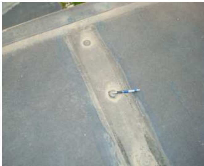
Same type of crack/cut at the covered fastener as noted on Roof Deck 1. All roof sections had this condition at various locations.
