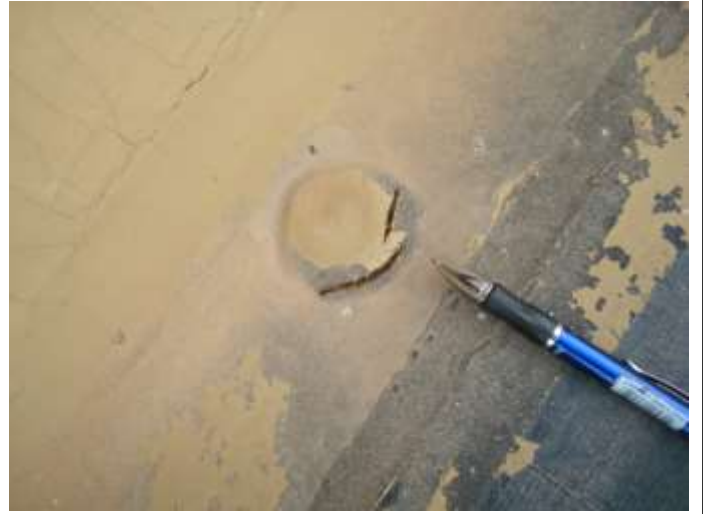
A little more pronounced cut/crack. This IS an area where a cut was made into the roof deck to determine if water intrusion has caused problems.
