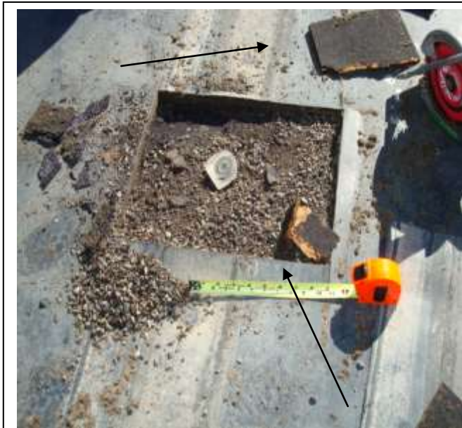
Roof deck 3. Directly under the EPDM is a black underlayment that looks like a “celo-tex” material with a 3/8” gravel below. The underlayment material is identified by the arrows.
