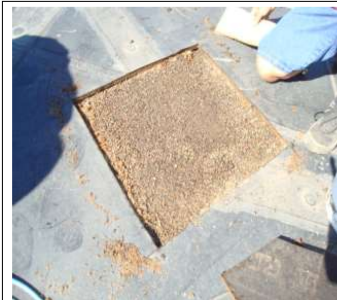
Roof deck 1. Underlayment was wet as was the gravel.
