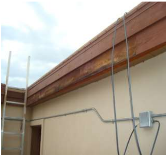
Weathered fascia and trim. Re-staining should happen soon.
