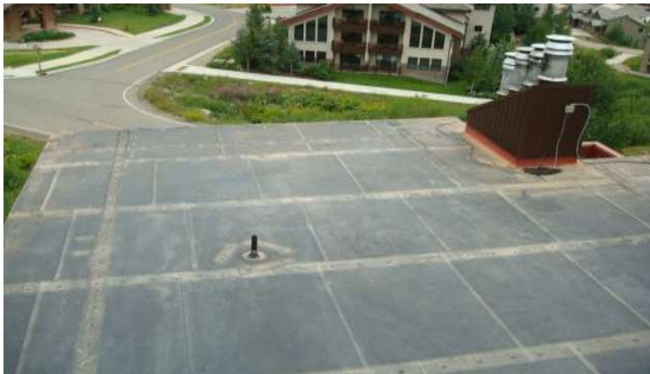
Roof Deck 4 exhibited similar small cracks as other roof decks.
