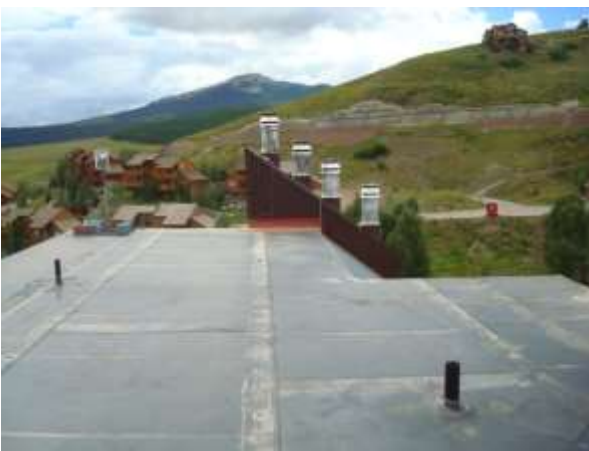
Roof Deck 1 overall photo. Photo depicts seams in the EPDM single ply roofing material, two of the three plumbing vents and the wireless LAN access point in the upper left corner.
