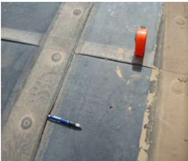
Photo shows loose seams between EPDM. To avoid further damage these seams were not probed. They should not be loose.
